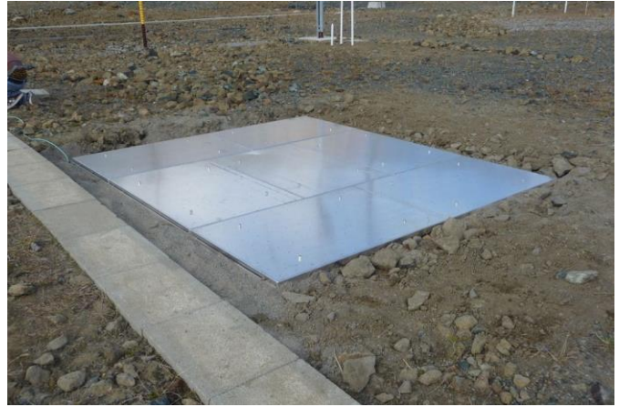
Figure 4: Installed SSG snow scale
